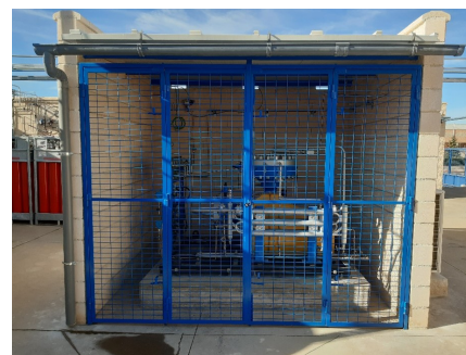
Figure 5: The hydrogen compressor placed in its location at CNH2 (Spain)
